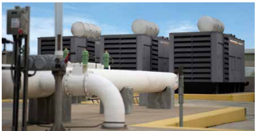
Generac Industrial Power 3 x 1000 kW Modular Power System (MPS)
