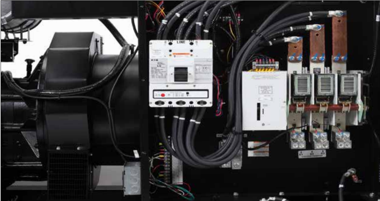
Paralleling Switching Device located on the generator.
