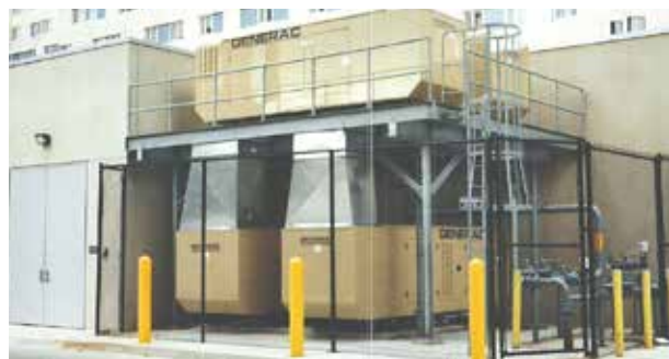
4 Generac generators stacked to meet tight footprint requirements.
