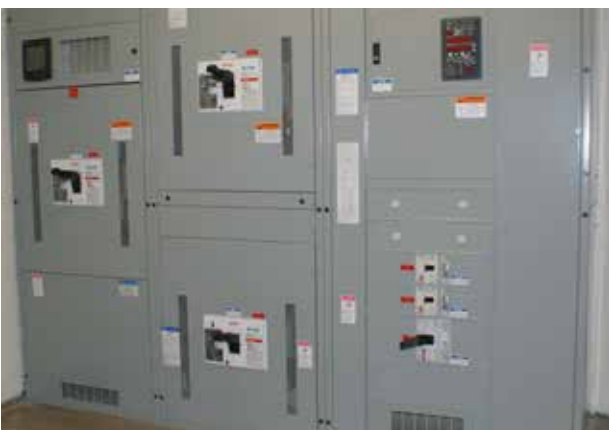
Traditional switchgear line-up with multiple generators.
